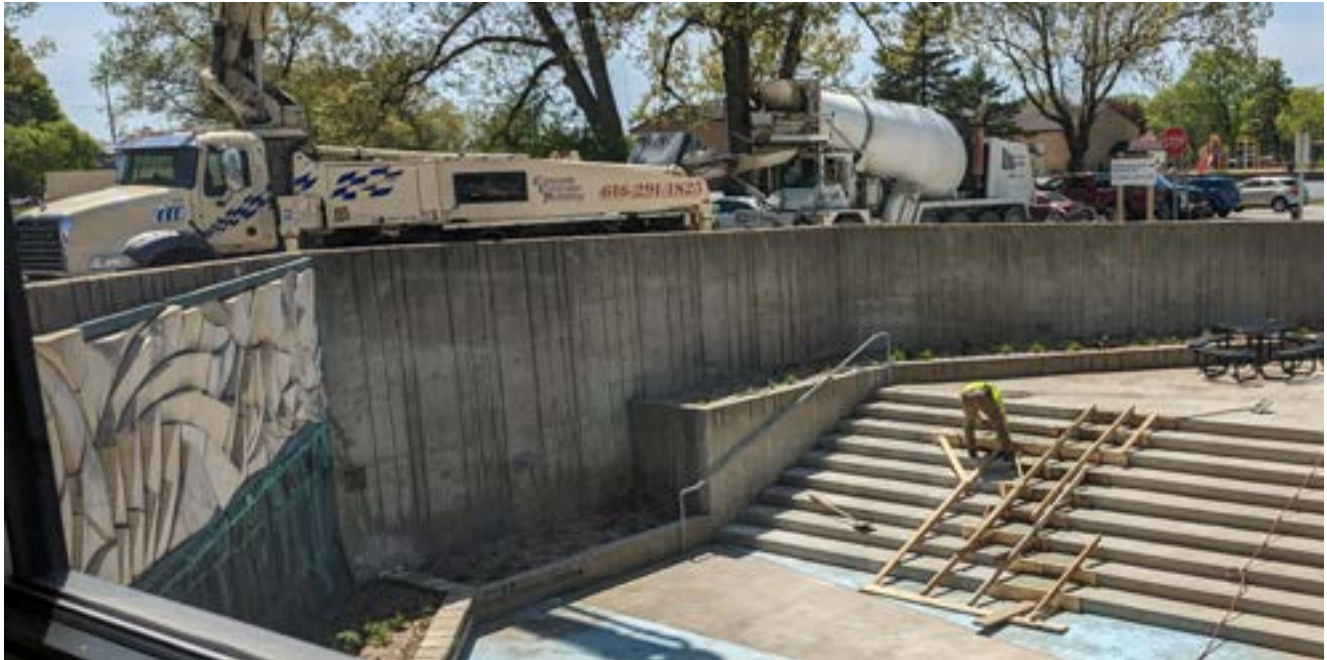
Concrete Pump Truck and Concrete Delivery Truck present for the replacement work on the courtyard stairs.
